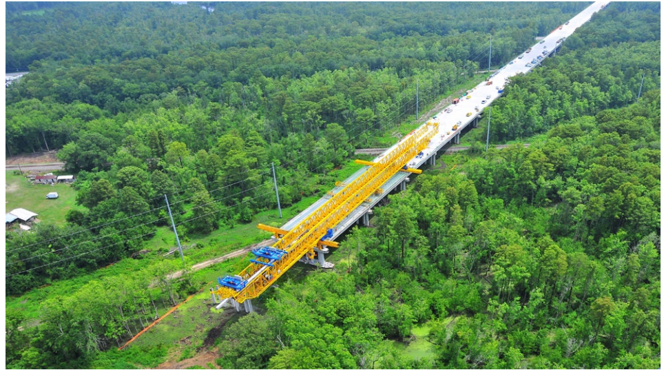
View of south end of bridge on US 17 over Tar River. More than 80% of the bridge (2.3 miles) is on tangent horizontal alignment with a continuous 70-ft. deck width (carrying four lanes of traffic), thus providing ideal repetitive conditions for this construction gantry operation.
